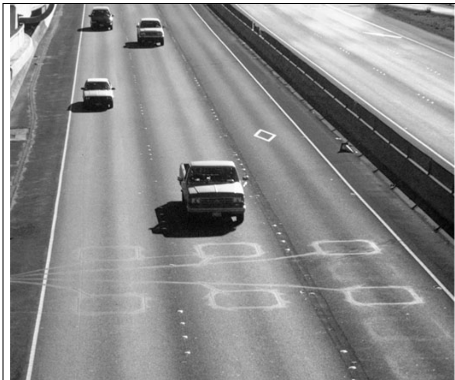
Pictured is a double loop detector installed on a California freeway. A single loop detector would look like just the top row.
